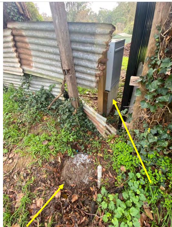
Main electricity pit with electricity box inside the site.
