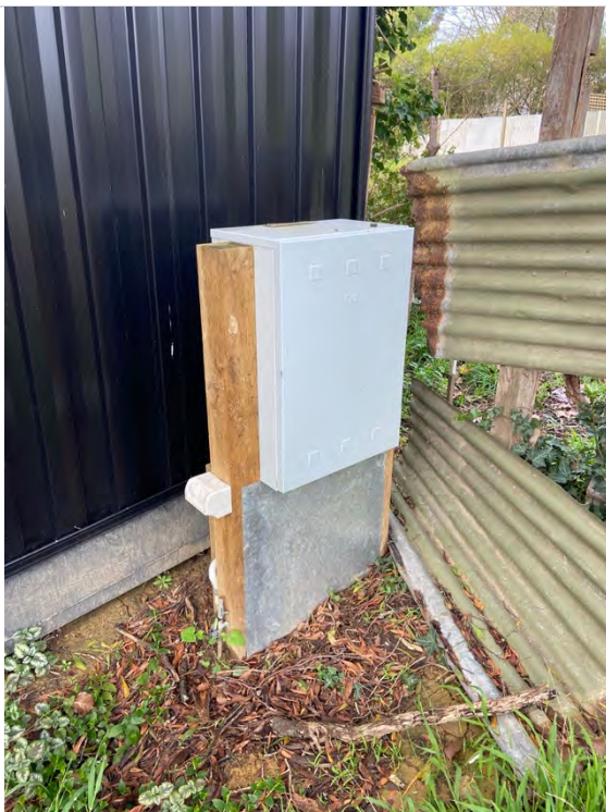
Electricity box in front corner of the site.
