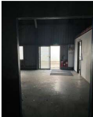
9. INSIDE WAREHOUSE 2 WHICH WILL BE OPEN ON THE EASTERN SIDE AND BECOME COVERED CAR STORAGE.
