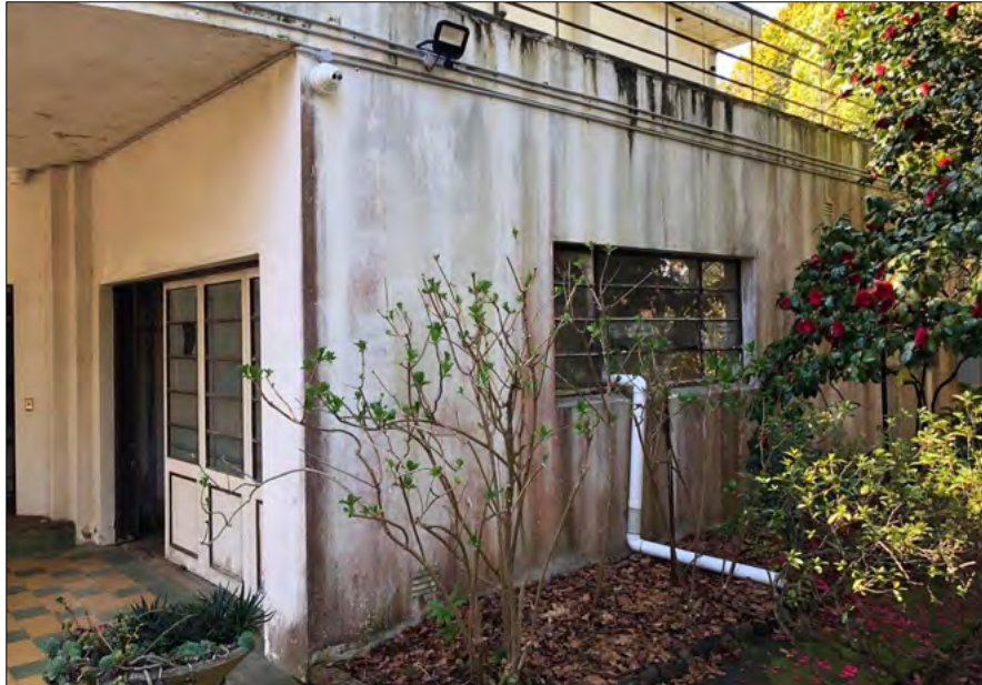
Figure 33 PVC downpipe directing water outside of the building from the first-floor balcony above.
