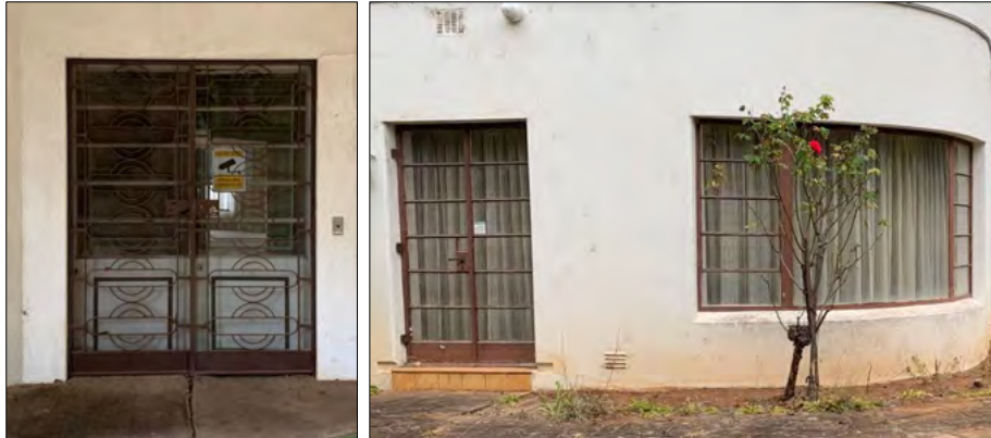
Figure 28 (left) Detail of the existing steel flywire doors to be retained and restored. Figure 29 (right) Detail of the existing steel windows and doors to be replaced to match the existing.
