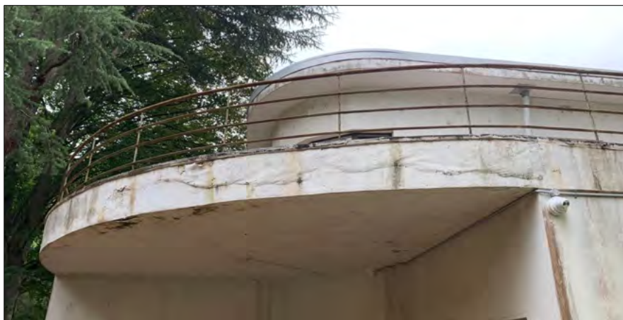
Figure 18 Detail of moisture damage to the render from first floor water egress.
