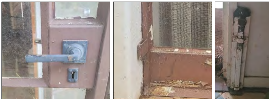
Figure 27 Detail of the existing steel door hardware to be retained and restored or recast to match the existing details.
