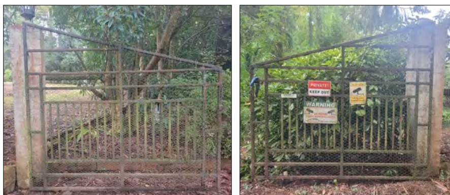
Figure 35 Existing southeast corner 'main' entry gates. Missing light from the right-side pillar to be replaced to match the existing light on the left side pillar.
