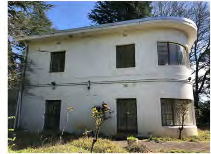
EXISTING CONDITION OF DWELLING
