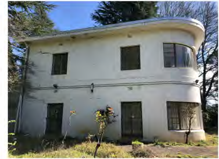
EXISTING CONDITION OF DWELLING
