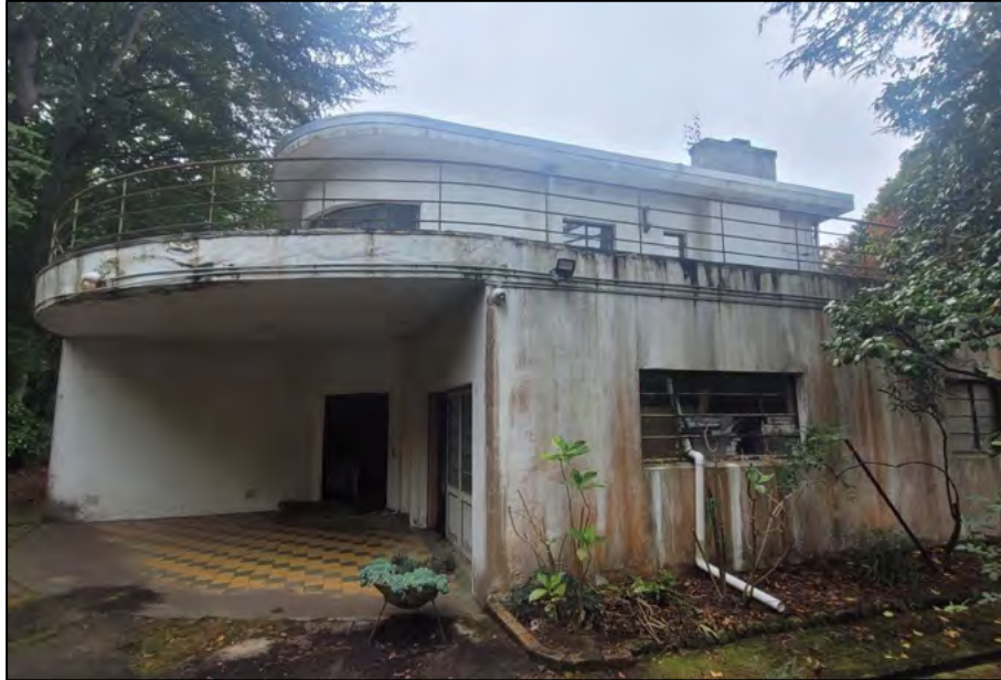
Figure 5 Portion of the south elevation, showing the weathered render and a glimpse of the chimney.
