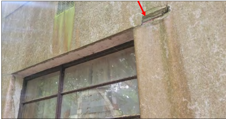
Figure 16 Detail of the existing upper corners of the window openings showing damage assumed to be due to corrosion of the associated lintel.
