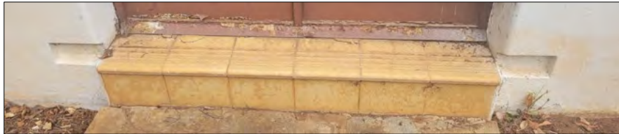
Figure 22 Detail of the existing typical tiled door sills to be retained and repointed.
