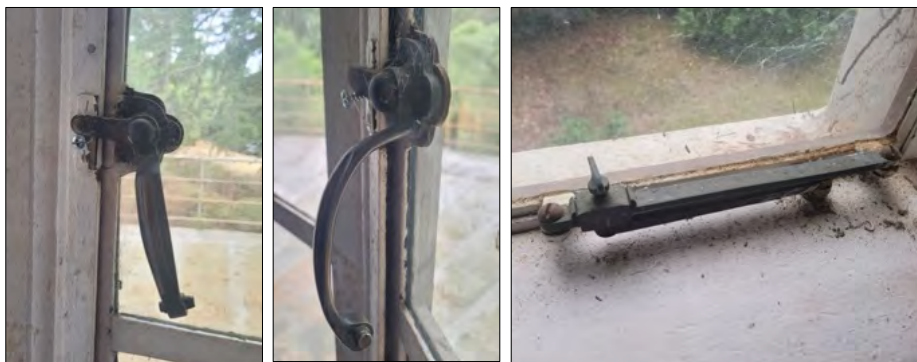
Figure 26 Detail of the existing steel windows hardware to be retained and restored or recast to match the existing details.
