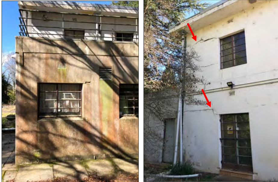
Figure 17 Detail of various render damage/repairs as indicated by red arrow.
