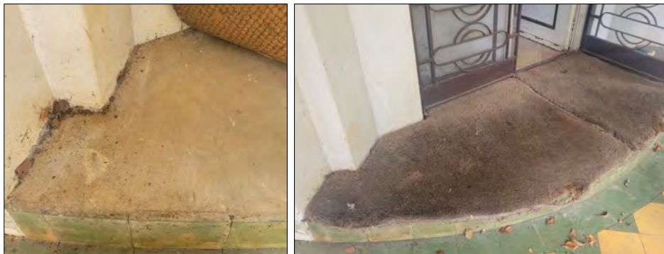
Figure 24 (left) Detail of the existing entry step with tiled edge and concrete below.
