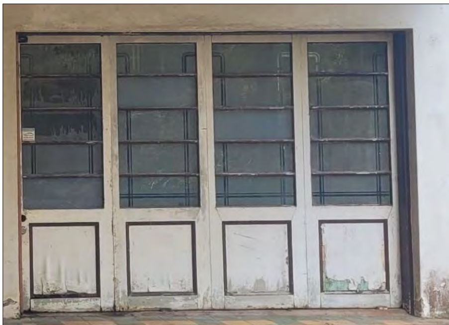
Figure 30 Detail of the existing timber bifold door to be replaced to match the existing.
