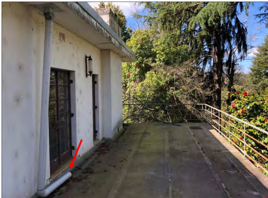
Figure 32 Detail of the first-floor balcony water egress. The existing spoon drain to the right (along the building wall line) is not effective enough in draining the water.
