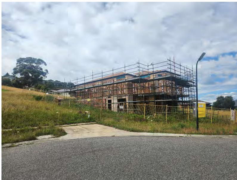
Figure 3: Lot No. 146 similar style of double storey home currently under construction. Photography taken 28/11/2024 via a Samsung Phone.
