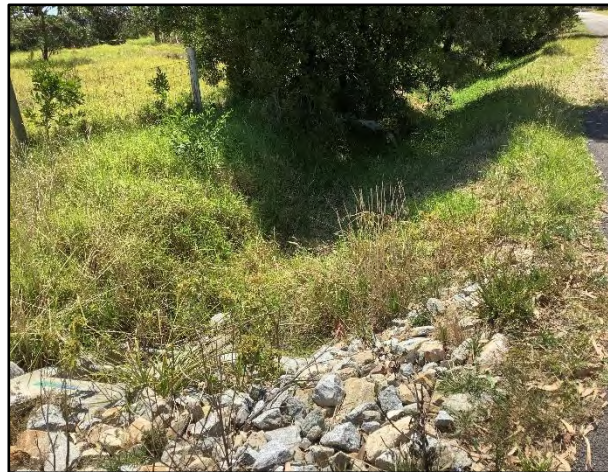
Photograph 3: Aquatic habitat – constructed drainage line devoid of fringing, emergent and floating vegetation.
