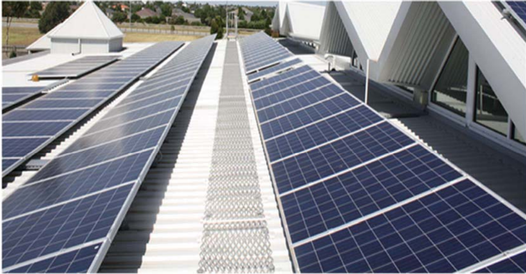
Figure 6. Arena Family and Child Centre solar electricity system
