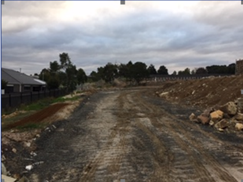
Figure 5. Mulcahy Road looking west to Moritz Street from Pointer Drive- soon to be constructed by developer
