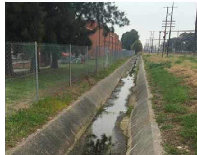
Open drain on railway reserve, located behind Pakenham Place
