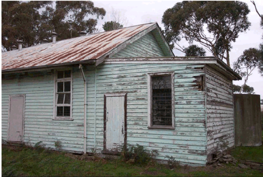
Figure 2 added rear skillion could be replaced or removed, given poor repair
